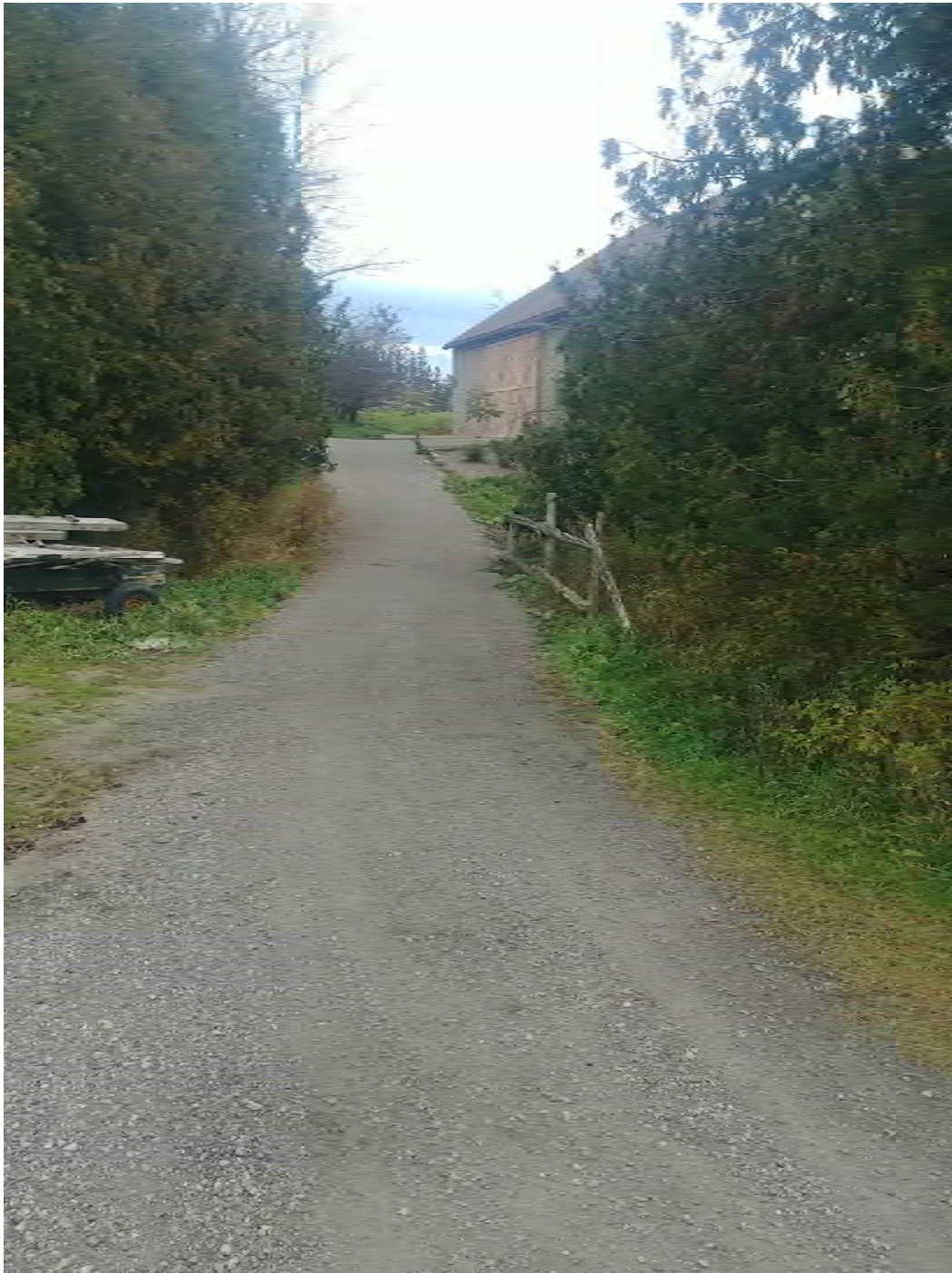
Photo 1. Existing driveway culvert crossing of watercourse. The driveway will not be altered.
