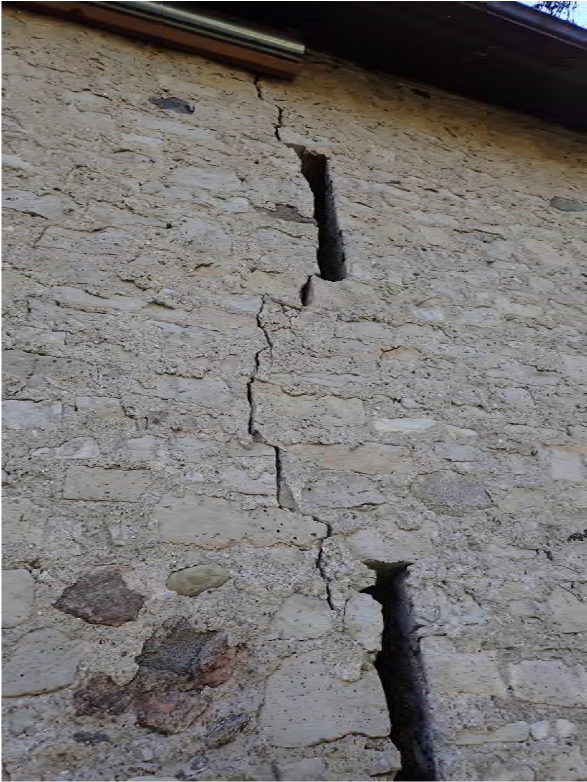
Photo 6. Example of cracking in stone walls. 'Slit' windows are shown.
