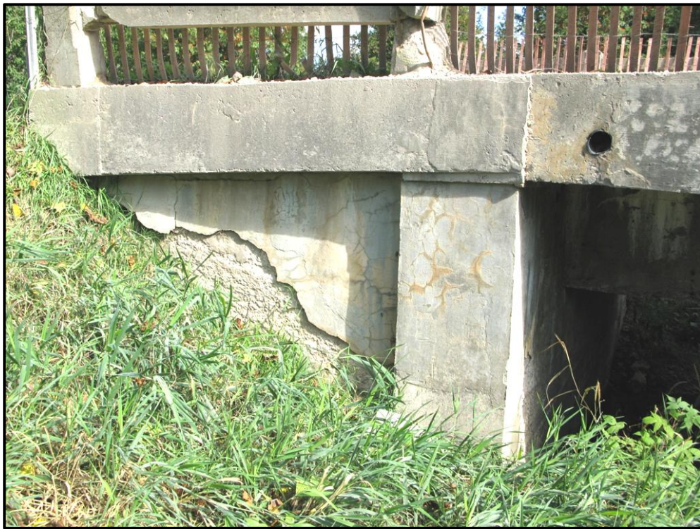
Plate 3: Detail of north abutment and west inset wing wall. Note spalling concrete resurfacing.
