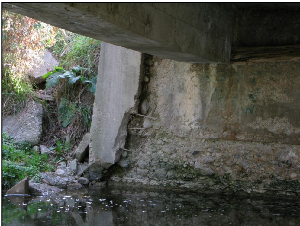
Plate 5: Detail of south east wing wall separation from south abutment. Note limited reinforcement and large cobbles.
