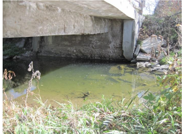
Photograph 14 ↑ Bridge structure – downstream side view of pool and debris along right bank
