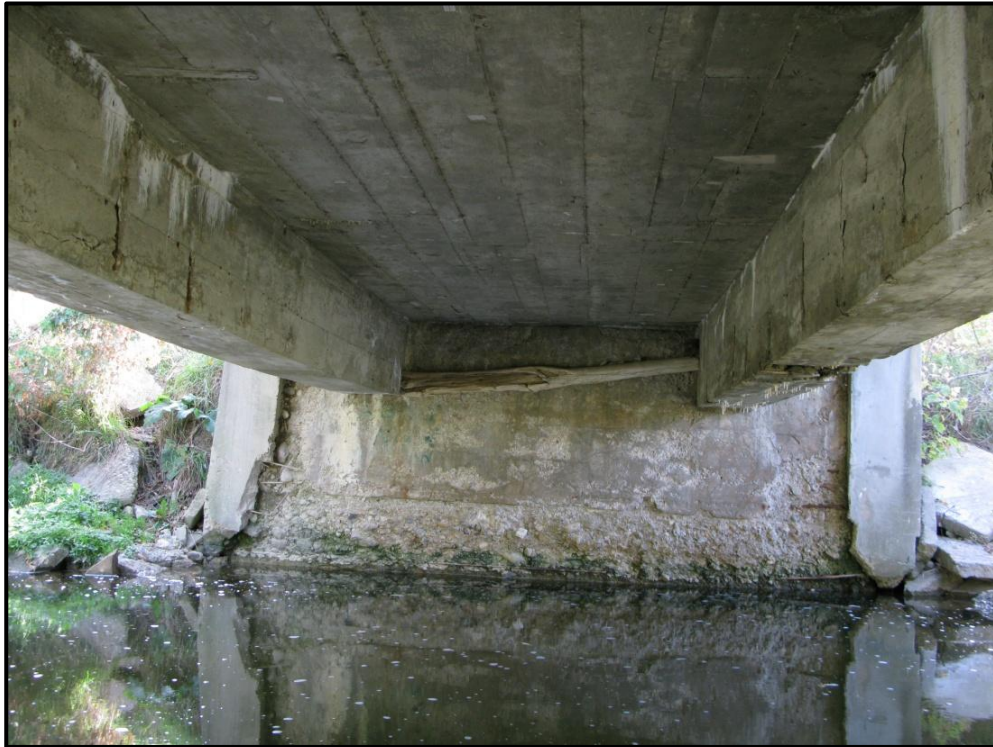
Plate 4: Carroll Creek bridge, south abutment showing "T" beams and deck bottom. Note new(er) wing wall castings separating from abutment and relatively clean edges of "T" beams.
