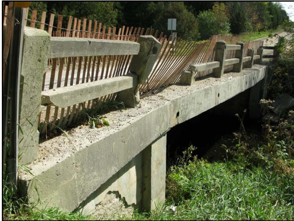
Plate 8: West deck edge showing relatively clean surface, but significant rail deterioration possibly due to collisions.
