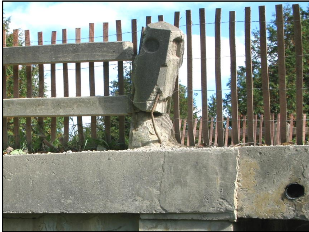
Plate 11: Failed balustrade and missing rails from west side railing.
