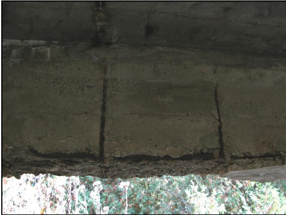
Plate 7: Detail of east "T" beam showing exposed reinforcement in lower beam half and connecting reinforcement integrating the beam into the bridge deck. Note missing concrete from beam bottom likely from corroding reinforcement and spalling concrete.
