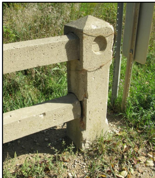
Plate 10: Balustrade detail of east rail showing pyramidal cap, chamfered edges, and decorative circular inset, and rail detail.
