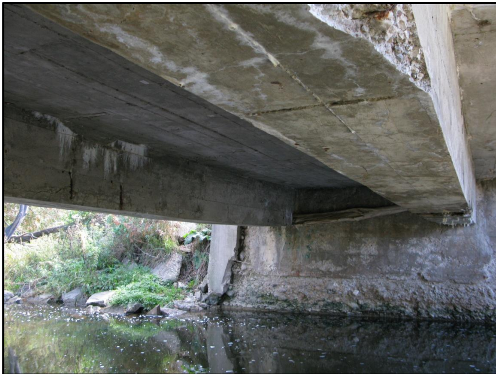
Plate 6: Two “T” beams and south abutment showing edge failures.
