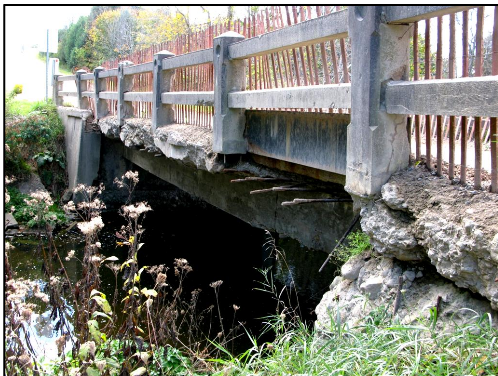
Plate 9: East deck edge showing significant deterioration likely due to ice and debris impacts during floods but relatively intact rail system.
