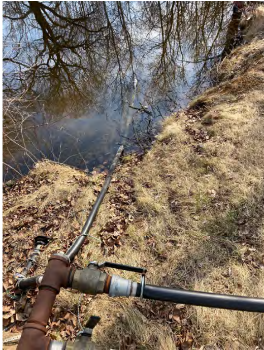
Photo 8 – Looking east behind the maintenance shed towards the unnamed pond showing water intake for turf irrigation.
