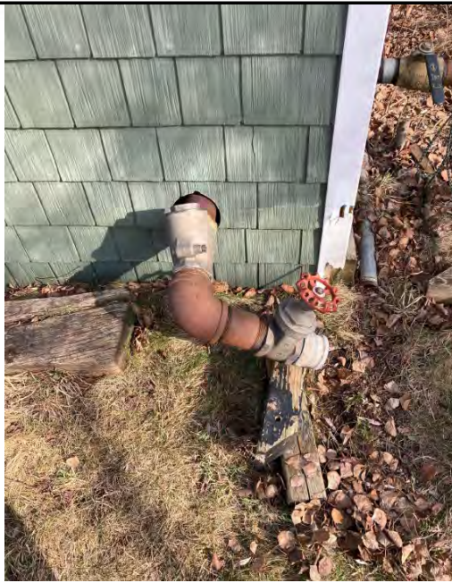
Photo 7 – Side of maintenance shed with pump for water intake for turf irrigation.
