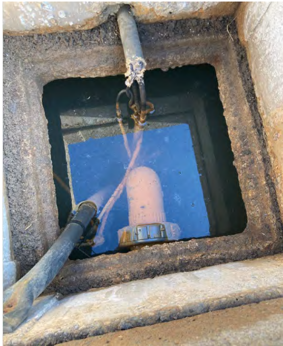
Photo 12 – Sump pump located in the front yard near the driveway, approximately 2 to 3 metres from the residence.
