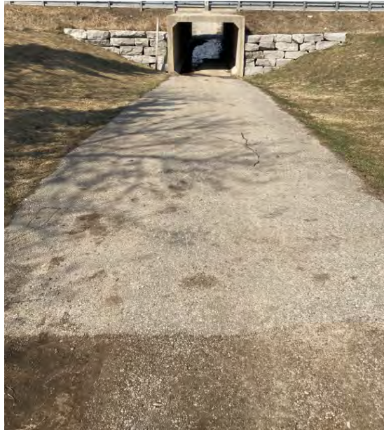
Photo 9 – Looking west towards the tunnel under Wellington Road 19 on the northwest end of the Site.
