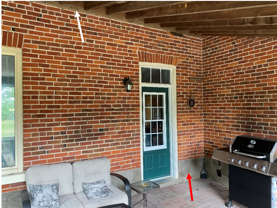
Photo 14: View of side door. Note canopy supported by the brick veneer (white arrow). Note cementitious parging over brick (red arrow).
