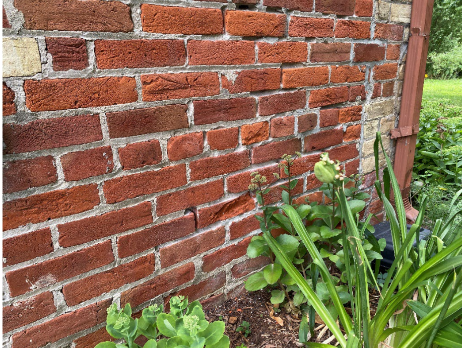
Photo 9: View of masonry deterioration. Note masonry extends below grade.
