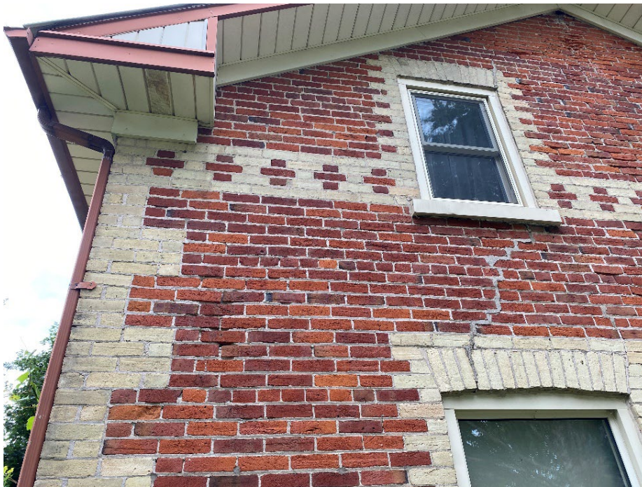
Photo 10: View of deteriorated brick.
