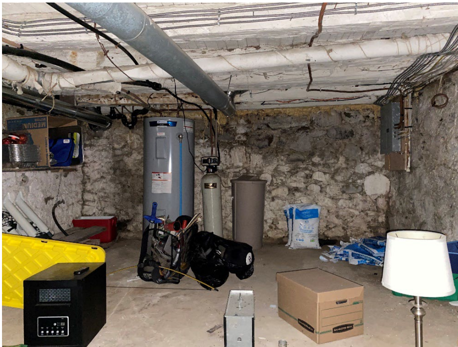
Photo 6: View of rubble wall foundation, note the extensive efflorescence.
