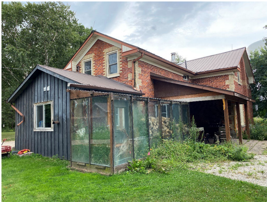
Photo 2: View of south west elevation, note the mudroom, greenhouse and canopy structures. Note canopy posts extend below grade.
