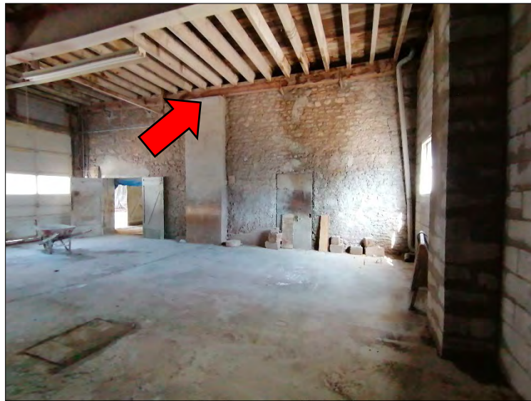
Figures 43 & 44: (above) View of north elevation of historic stone building (Building B) showing concrete carport and location of steel beams on this elevation; (below) View of attachment of western addition to historic stone building (Building B) (Source: MHBC, 2021).
