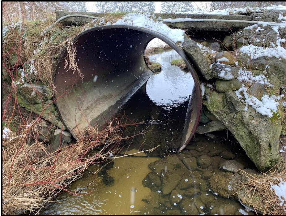
Photograph 1. Steel Pipe Culvert Under the Driveway to The Property. Facing Upstream (April 19, 2022)
