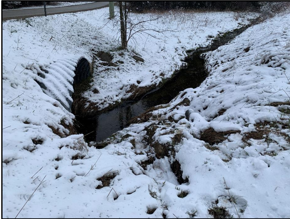
Photograph 7. Photo Taken From The Roadside Ditch Showing The 1.5 m Drop to The Watercourse (April 19, 2022)
