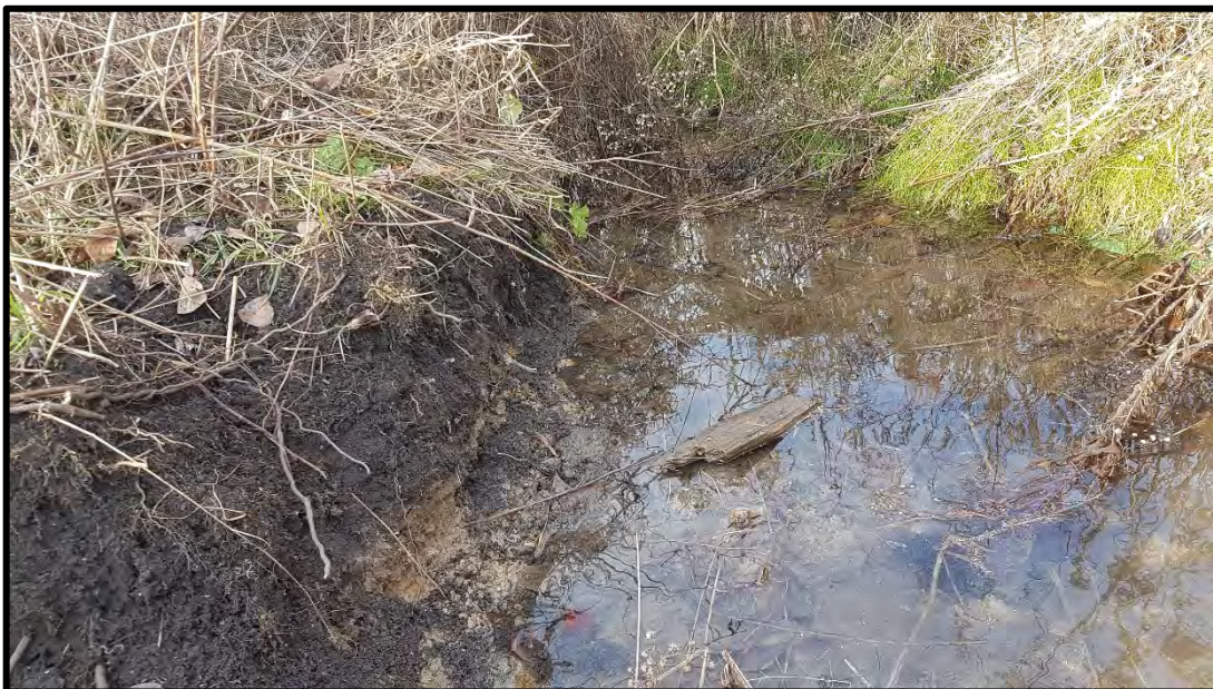
PHOTOGRAPH NO.: 6 FROM: Culvert LOOKING: Downstream NOTES: Scoured, soil banks
