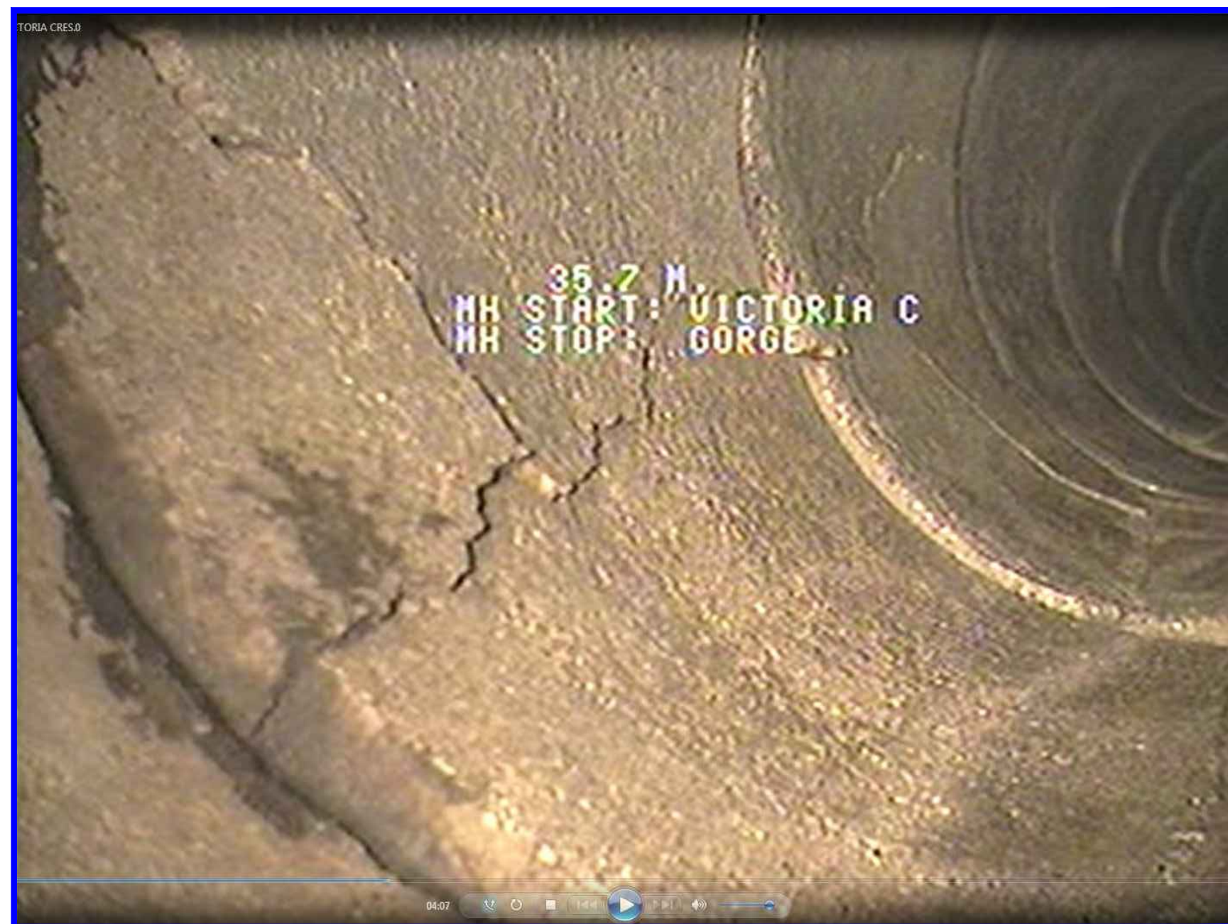
P4 June 2006. Long horizontal cracks in existing trunk storm sewer.
