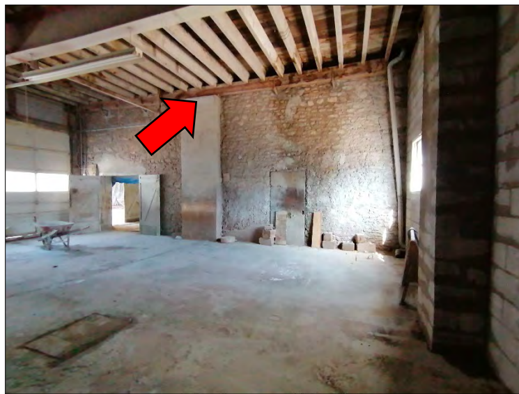
Figures 49 & 50: (above) View of north elevation of historic stone building (Building B) showing concrete carport and location of steel beams on this elevation; (below) View of attachment of western addition to historic stone building (Building B) (Source: MHBC, 2021).
